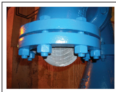
VentSafe® Security Cage Installed on Vent Pipe
